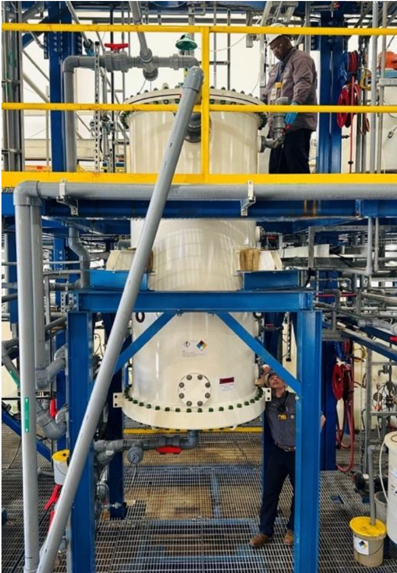
Figure 13-4: Commercial-Scale LSS Column at the Demonstration Plant
