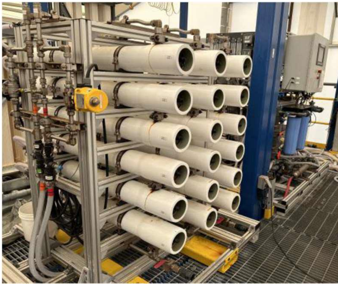
Figure 13-7: Osmotically Assisted Reverse-Osmosis System at the Demonstration Plant
